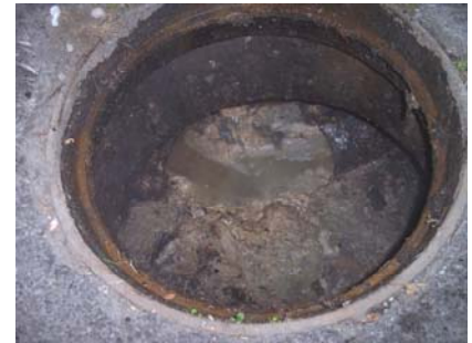
Sewer line blockage from grease.
